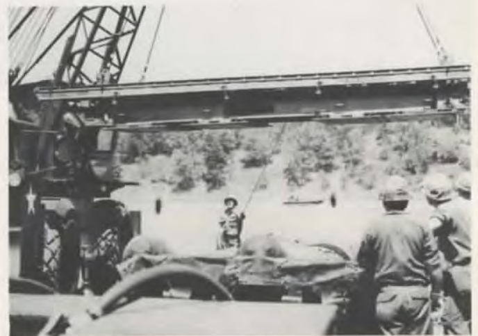
47th Division Engineers construct a bridge across the Mississippi River; mobility is their primary mission
