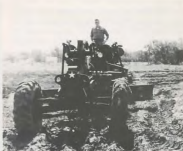
An Army Guard grader constructs a new parking lot at the Gibbs Farm Museum
