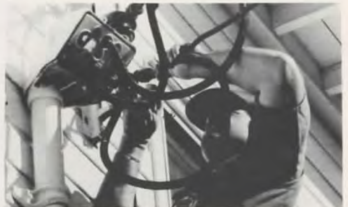
A member of the Minnesota Air Guard's 210th Electrical Installation Squadron repairs electrical wiring at a U.S. Air Force base. Such projects save taxpayers money while providing on-the-job experience for unit personnel
