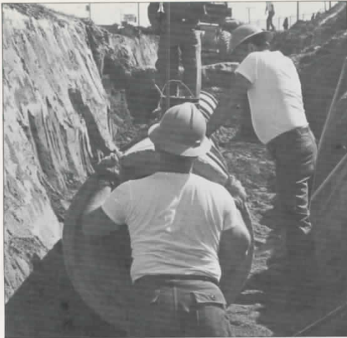
Air Guardsmen of the 133rd Civil Engineer Flight lay pipe at Luke AFB, Ariz., during annual training
