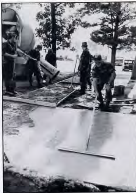
Company C, 142nd Engineers lay cement for a new sidewalk at Camp Ripley.
