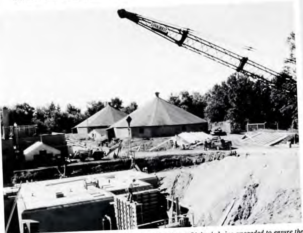
Built in the 1930's, the Wastewater Treatment Plant at Camp Ripley is being upgraded to ensure the operational excellence which earned a special Governor's Award in 1987.
