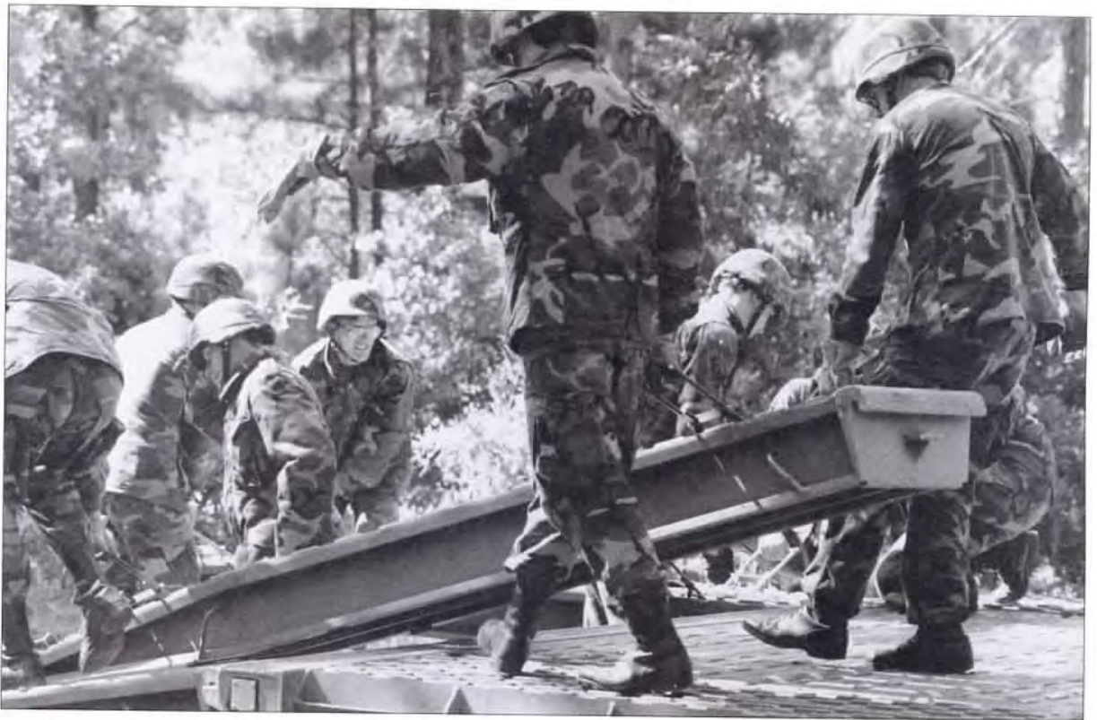
Members of the 682nd Engineers carry medium girder beams to build a bridge at their annual training.
